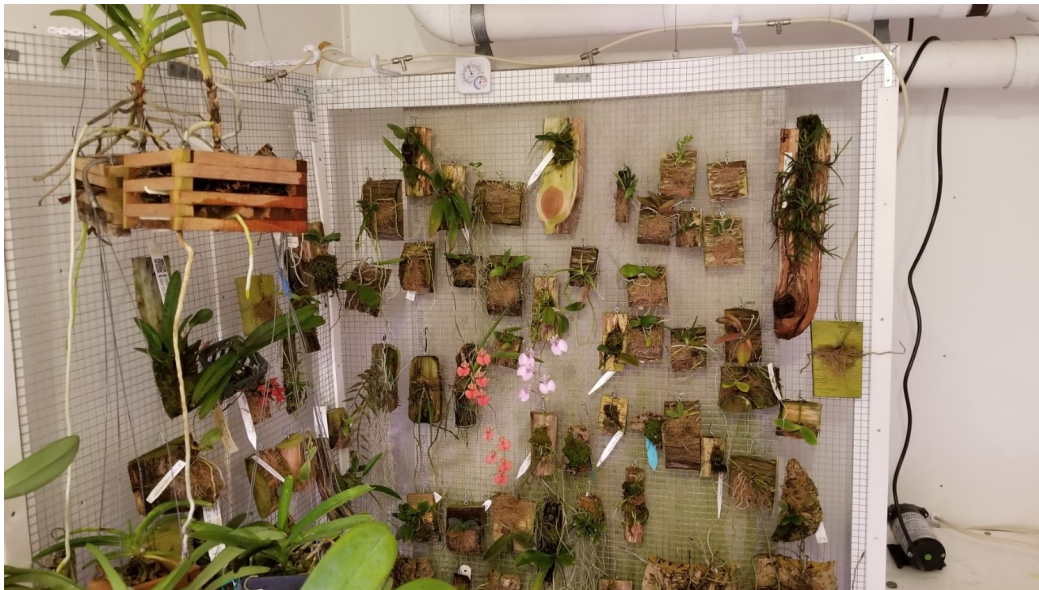
Mounted orchids with pump and misting system temporarily installed
